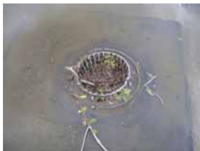
Figure 3. A severely clogged roof drain (the guard is up-side down).
