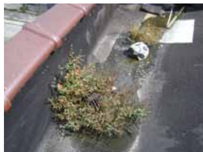
Figure 4. Vegetation grows around and inside this roof drain.
