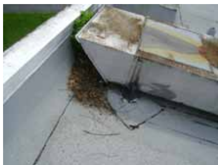
Figure 1. Vegetation grows under this HVAC ductwork.
