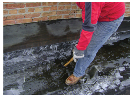
Figure 4. Water and ice cleared from a roof this past December.
